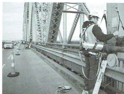
Figure 25.6 A worker is installing a strain gauge on a bridge to measure how much a part of the bridge is distorted when a load is put on it.
